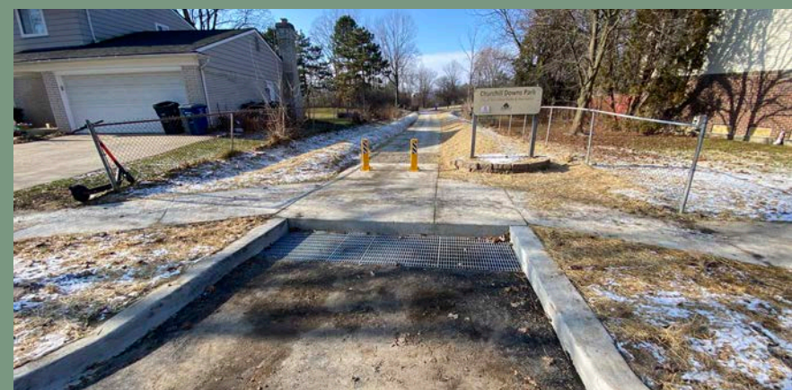
Top Photo - Inside of outlet control structure Bottom Photo - Downstream end of project, outlet control structure
