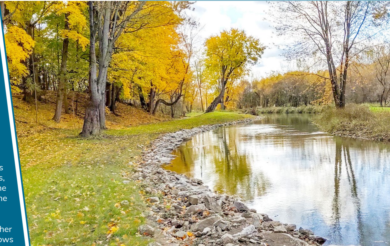
Post-construction view of the Swan Creek Intercounty Drain, with a maintenance lane created and riprap installed.
