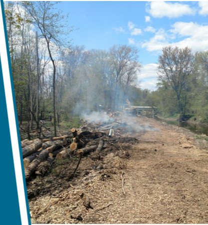
Trees were removed along the Swan Creek Drain to create a 20-foot-wide maintenance access lane.
