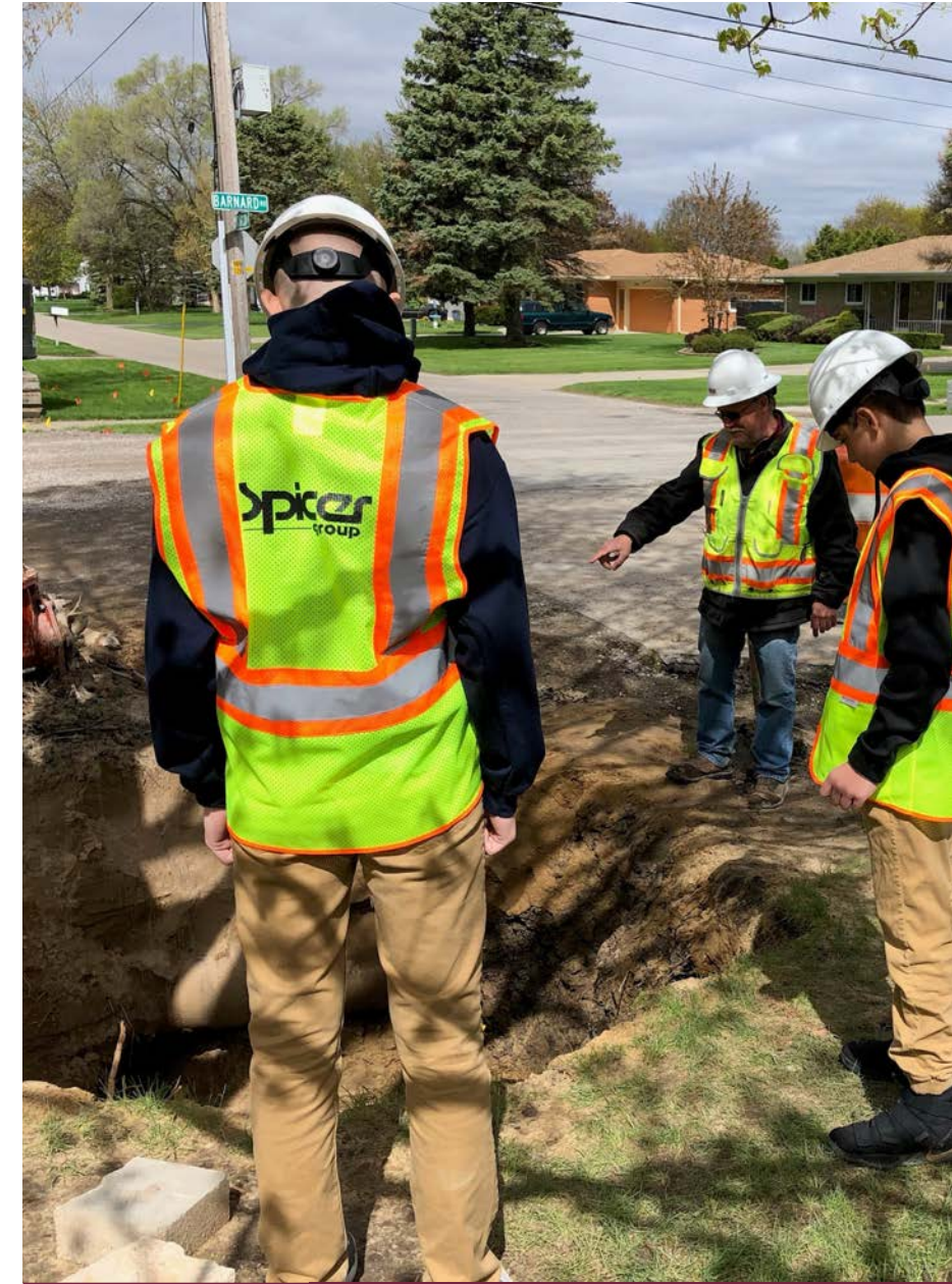
Spicer Group Construction Inspector Mark Goss takes a moment to explain to some 8th-grade students how a new water main is installed.
